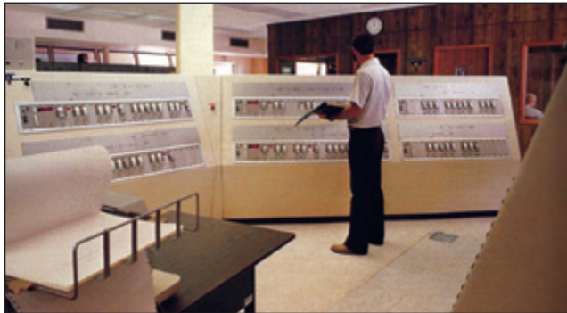
Figure 34. DYMAC monitors in an ammonia plant.
